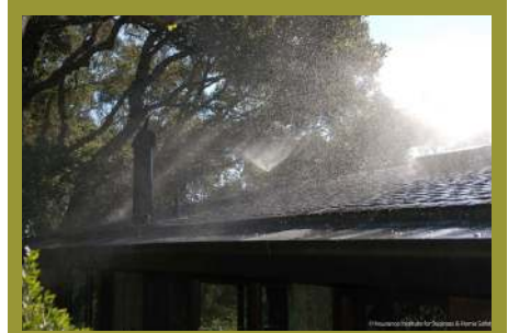
Photo 1. Roof mounted sprinkler.
